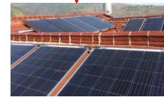
Hybrid solar thermal and photovoltaic panels
