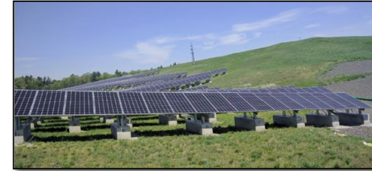
Example of our Landfill Solar Development
