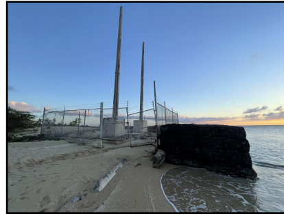
Figure 2. Exposed submarine cable
