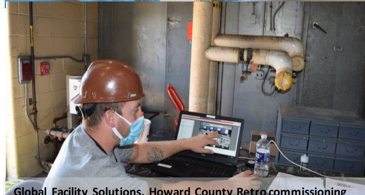
Global Facility Solutions, Howard County Retro commissioning
