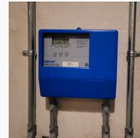
Figure 6: Old Boiler Controller
