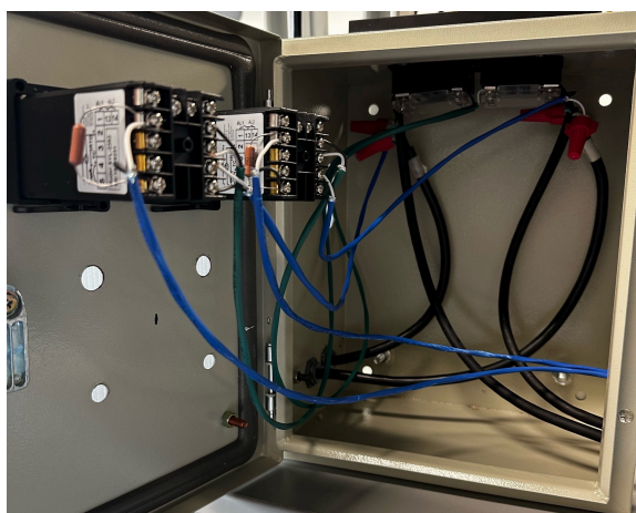
Figure 6: Temperature controller in the electrical junction box.
