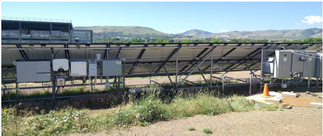
Figure 2: NREL's Outdoor Battery Test Facility in Golden, CO
