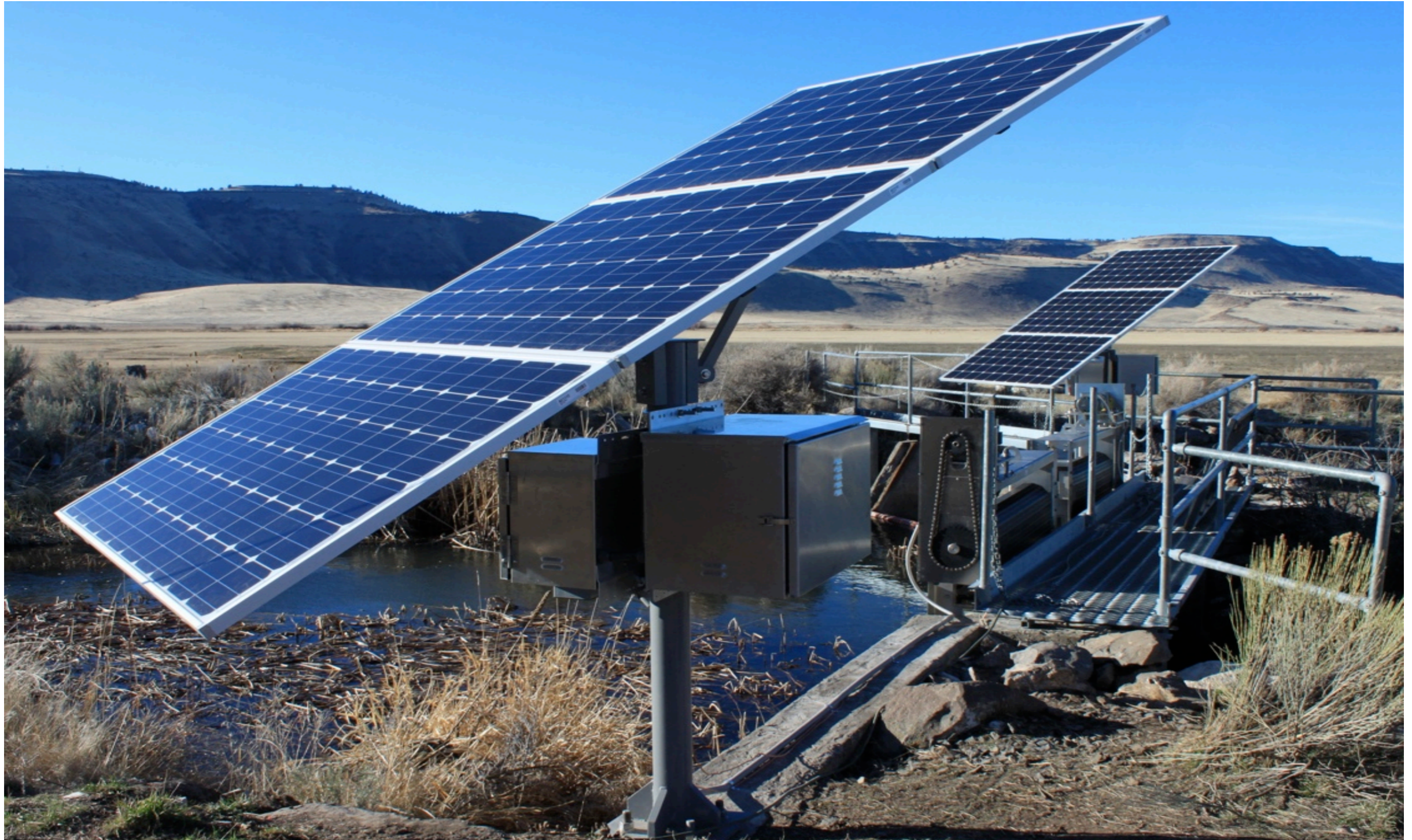
Ameristar Solar LLC, 1-5 KW Fixed Solar Panel Battery Charging Station U.S. Fish and Wildlife Service, Malheur National Wildlife Refuge
