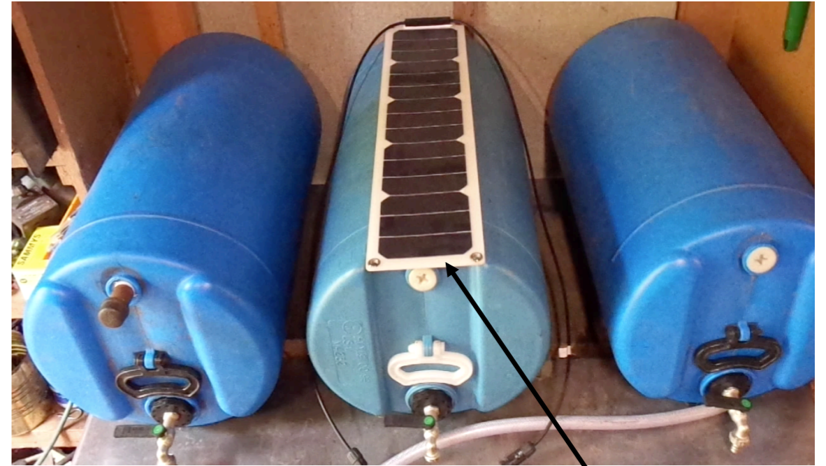
Solar Panels with UV Window
