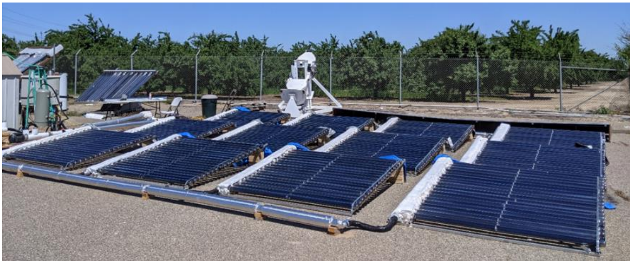
Figure 1 – 10kW ICPC array installed at UCM
